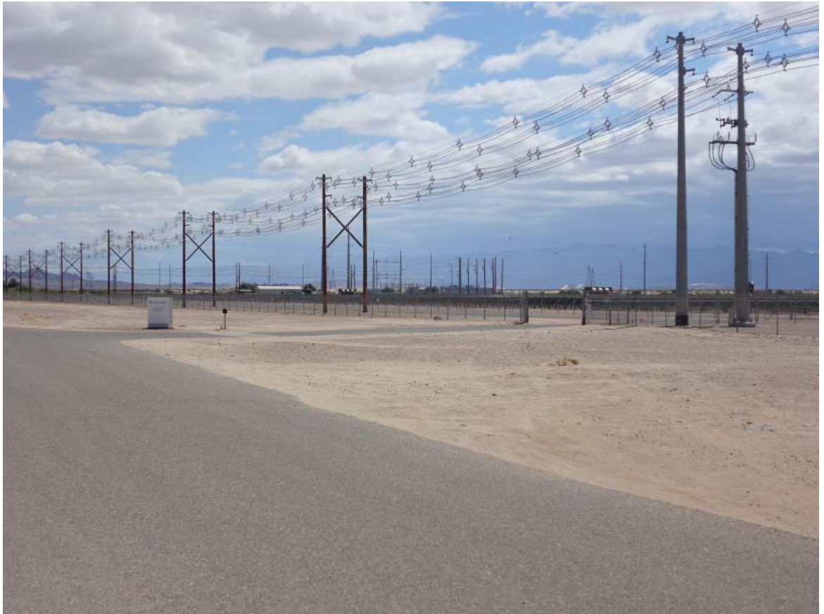
VP1 - View looking southwest toward the IID Campo Verde solar generation facility
