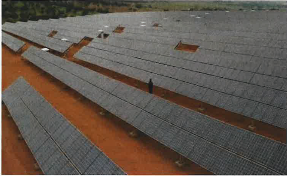
Typical fixed-tilt solar panel rows
