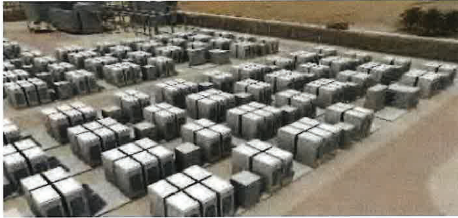
Modular BESS Installed on Multiple Concrete Pads
