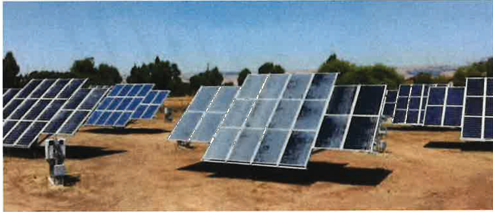
Typical dual axis tracking solar panels
