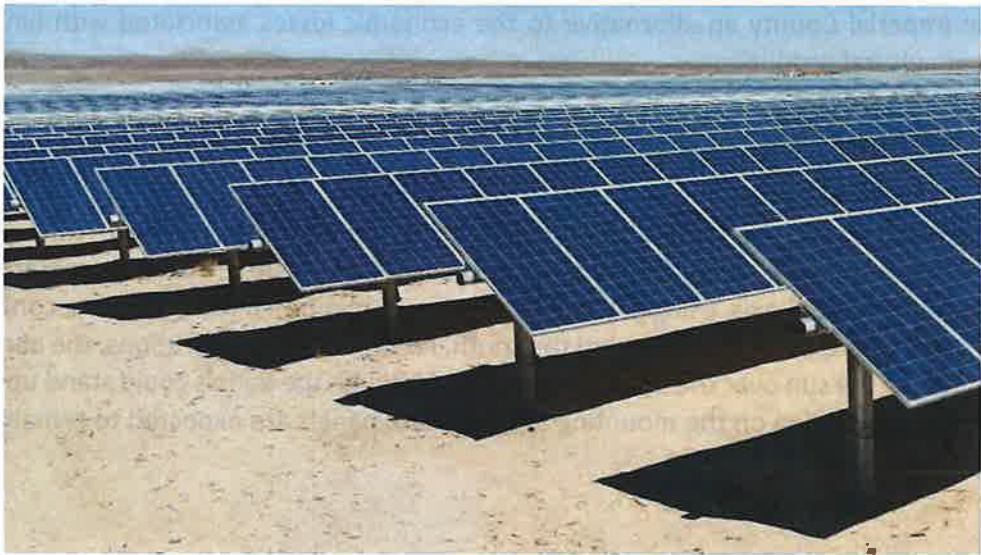
Typical single axis tracking solar panels
