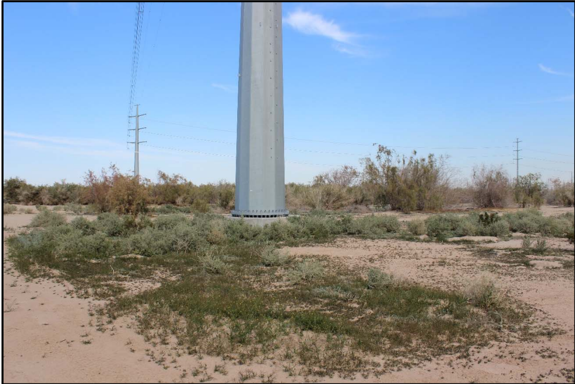
Photo 11: Large metal power pole in the northwest corner of subject property.
