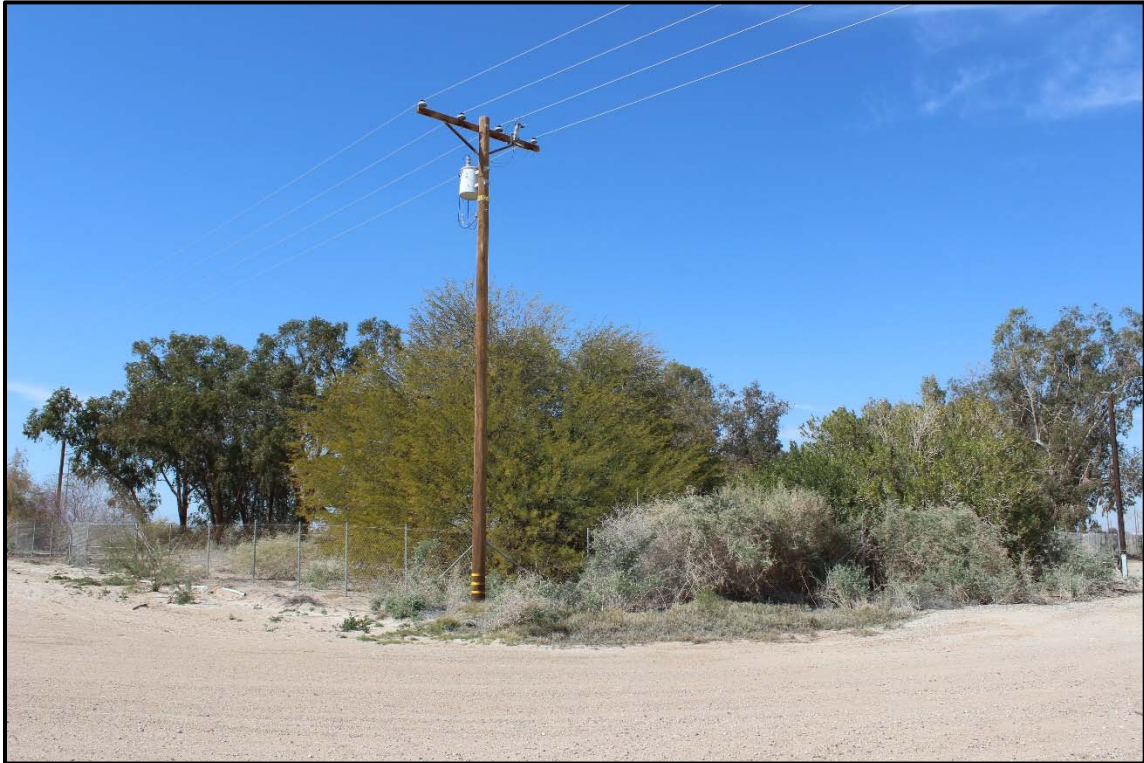
Photo 13: Pole mounted transformer in the northwest corner of Liebert Road and Westside Main Canal.
