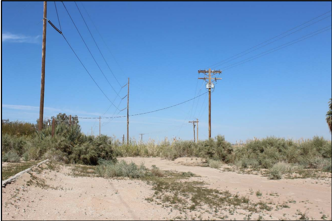
Photo 9: Pole mounted transformers in the northcentral portion of the subject property.
