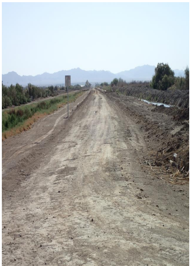
15. Alcott Road looking east; IID drain and canal: not BUOW foraging or burrowing habitat 15
