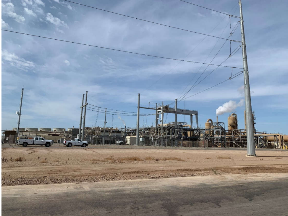
Photo 37: Looking at the Gen-Tie termination area of the existing power substation from McDonald Road.
