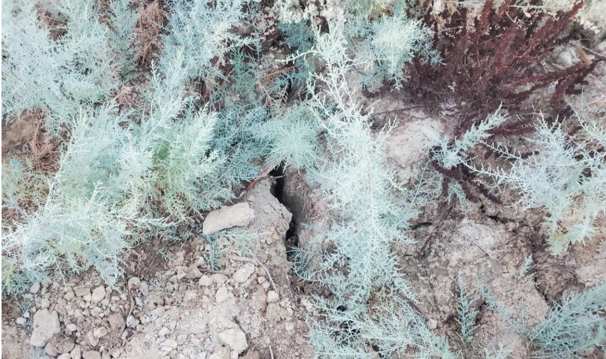
Photo 13: View of vegetation and surface soil cracks at WPF-7.
