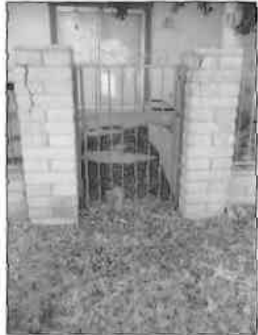
Location of MH 25 within a private patio, as located by the video camera with a tracking device.
