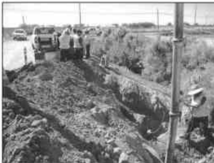
Second video inspection of the force main along Barbara Worth Drain, pump station is in the left background. The end of the pipeline can be seen in the trench, one line in the pipe is the video cable, the other is the jetter line used to pull the camera into the pipe.
