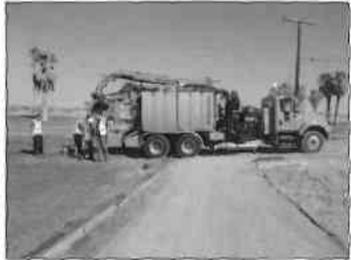
Vactor truck cleaning operations at newly located MH 7 within the golf course. Note the size of the equipment required to efficiently maintain the system.
