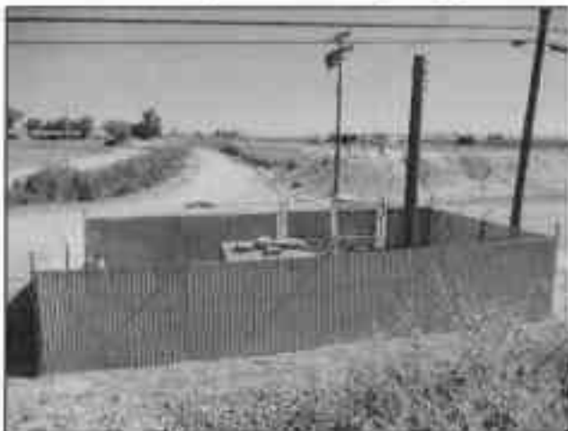
Wastewater pump station
