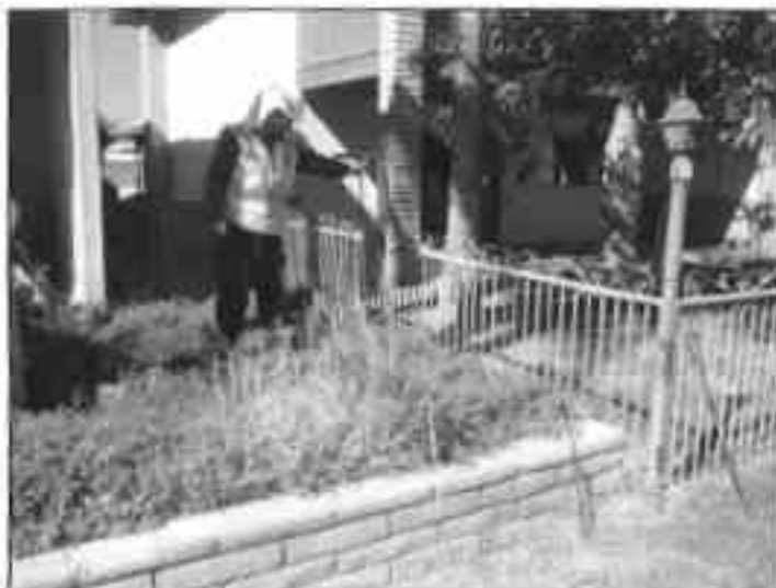
The worker is holding the probe at the center of MH 29, which is in a private backyard underneath the decorative wall on the left and the wrought iron fence on the right.
