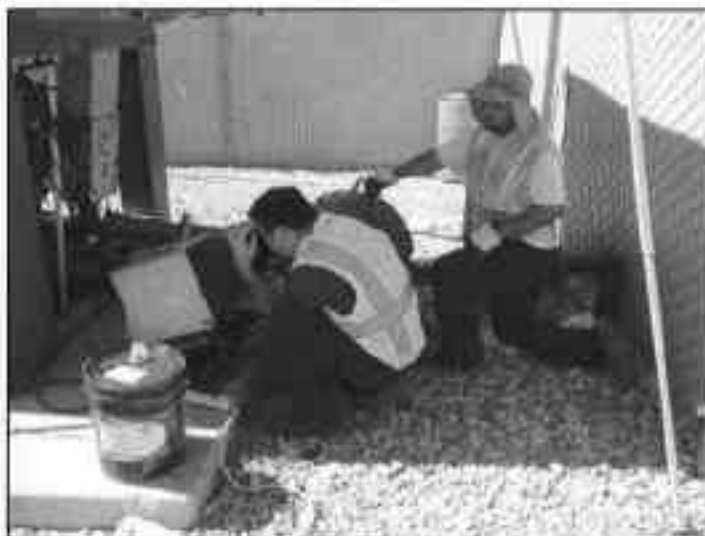
Initial video inspection of the force main with a push camera. Pump station is on the left and force main is on the right. Note the sharp 90-degree bend in the force main next to the fence.
