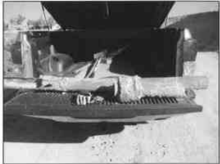
Existing 4-inch force main pipe removed from the trench. Note the splintered section on the left, repair coupling in the middle, and the barely visible chip and crack in the spigot end of the shorter section on the right.
