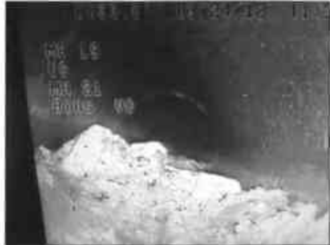
Image taken directly from CCTV camera shows an 8-inch pipeline between MH 19 and 21 that is 25%+ full of silt and debris.
