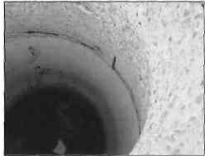
Manhole 5 showing corrosion.
