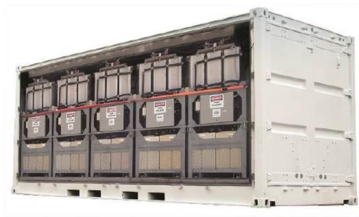
Figure 2-6. Representative Example of Battery Energy Storage Systems
