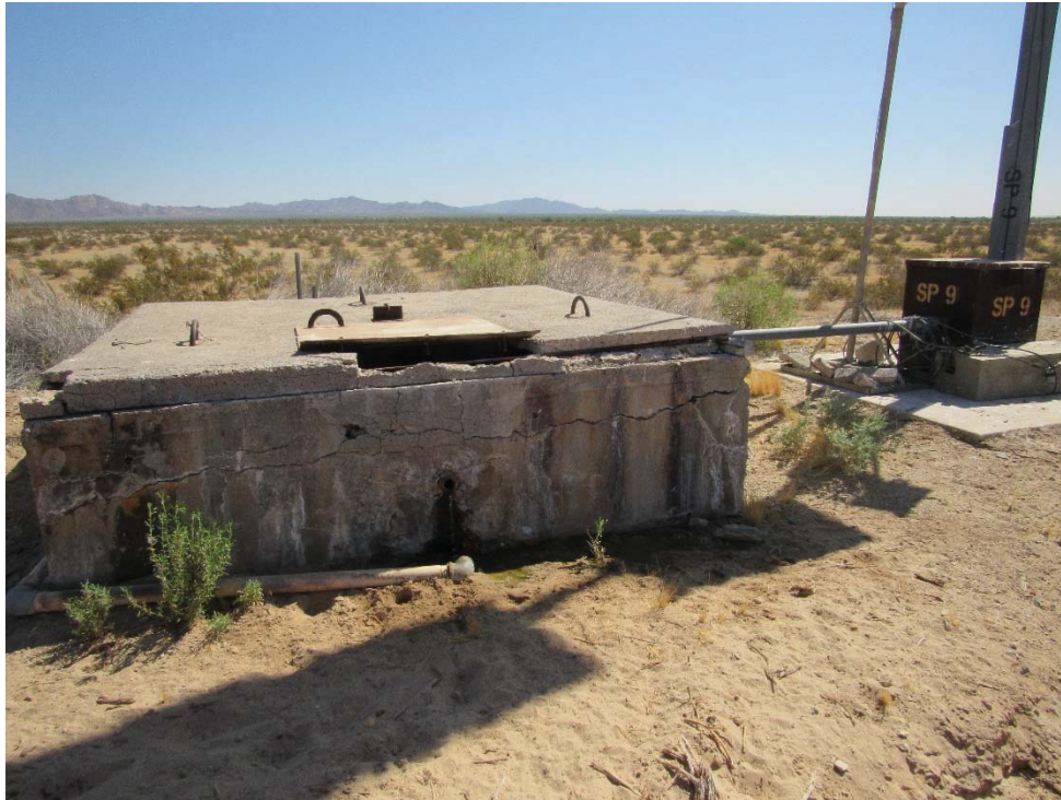
Photo 36: Looking at a wildlife water drinker (SP-9) located east of the Coachella Canal near the siphon within the subject site.
