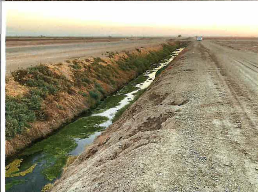
Photo #2 Burrows observed on the north bank of the Magnolia Drain.
