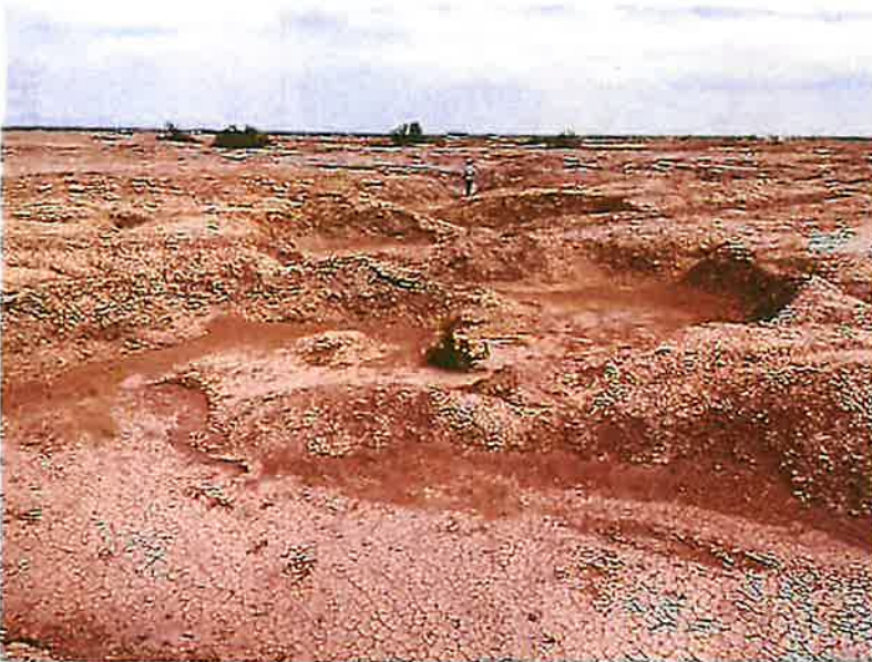
Photo 2: Drainage 1 where a bed, bank, and channel begin to develop within the Impact Area of proposed well pad 18-32 (at RA 1D) after being partially diverted by Drainage 2 at RA 2. Photo taken facing east along the southern edge of the access road Impact Area on April 26, 2022.
