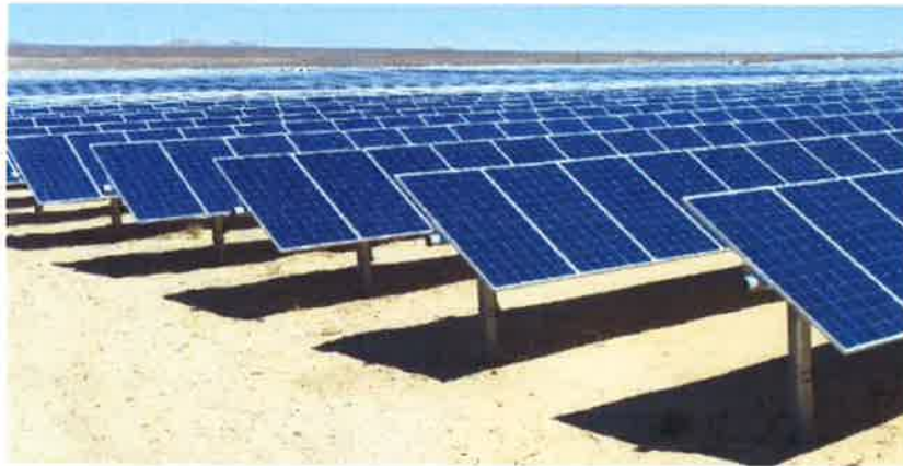
Typical Single-Axis Tracking Solar Panels
