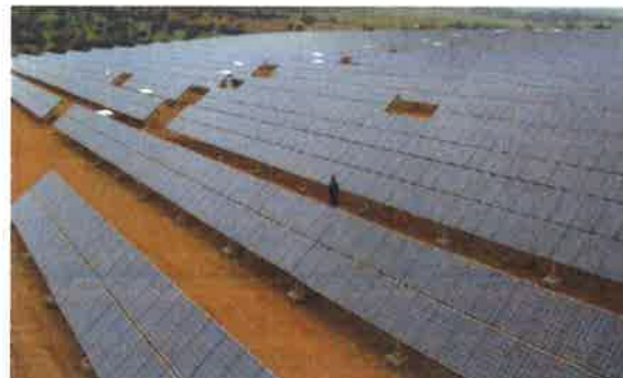
Typical Fixed-Tilt Solar Panel Rows
