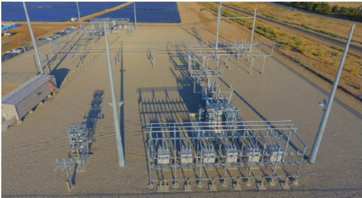
Figure 6. Representative Example of Typical Substation Design
