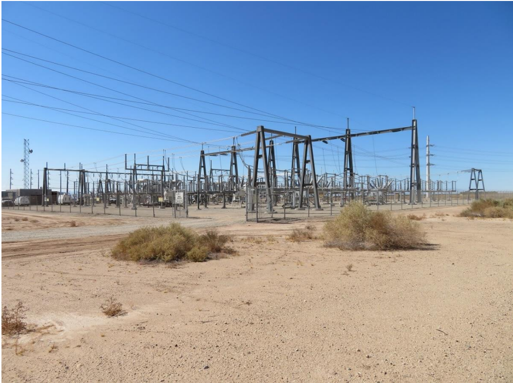
Photo 7: West-facing view of the Midway Substation.
