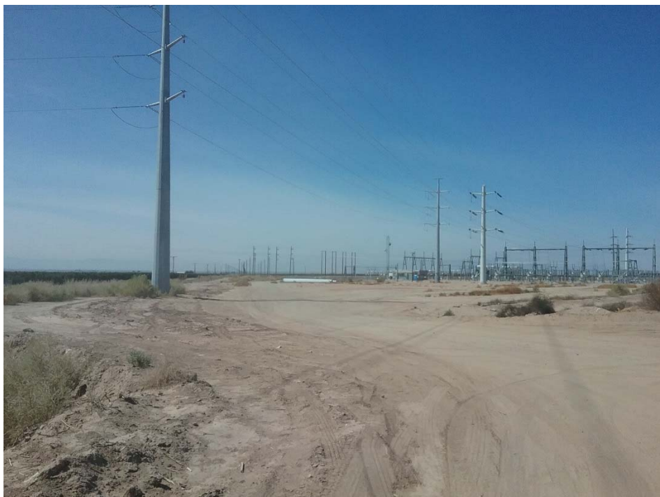
Photo 2: Looking west at the IID substation from the southeast corner of the north parcel.
