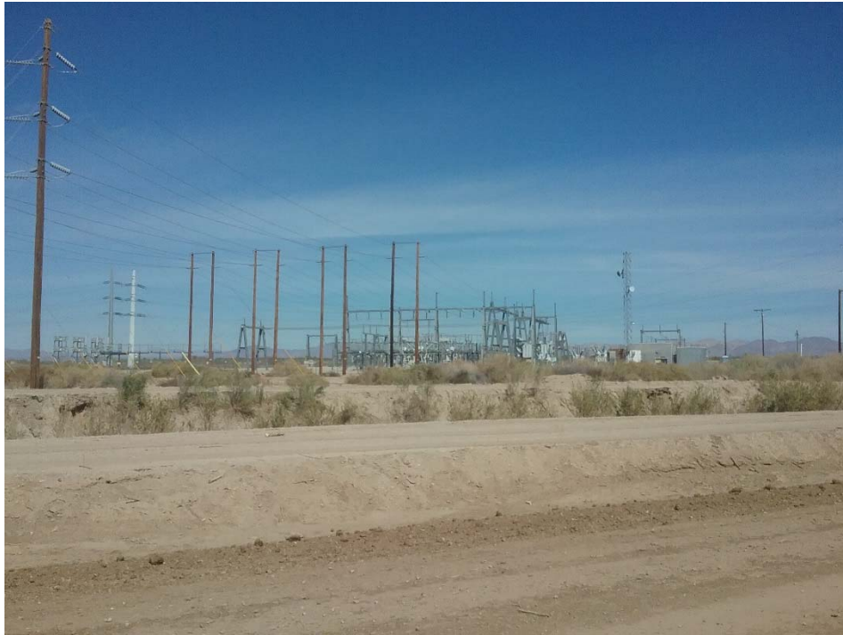
Photo 1: Looking north at the IID substation from the southeast corner of the north parcel of the subject property.
