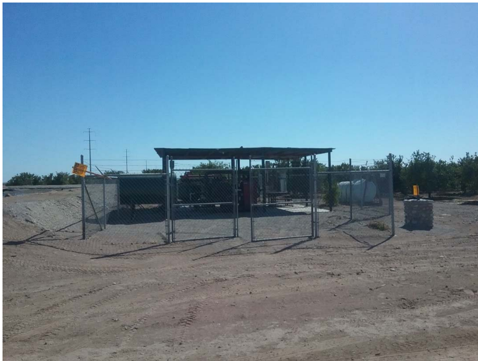
Photo 22: Looking at the neighboring P&T Enterprises irrigation reservoir diesel pumps and above ground diesel tank located west of the northwest corner of the southern parcel.
