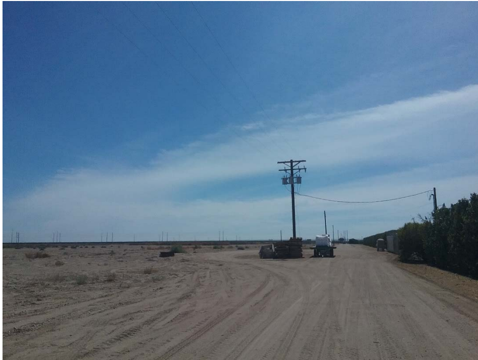
Photo 7: Looking south at the pole mounted transformers along the west boundary of the north parcel.
