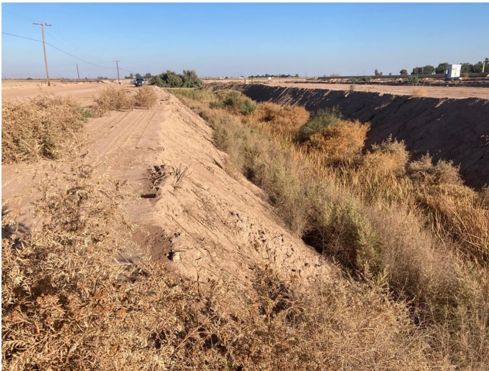
Photo 2. Photo of the eastern end of the Spruce Three Drain, forested shrub wetland, jurisdictional feature. The vegetation community consists of Riparian scrub. Photo facing east.
