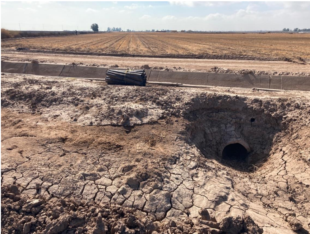
Photo 12. Photo of a culvert that is in the center of the north side of the Project site. It is surrounded by mainly bare ground with man-made ditches running through. Photo is facing north.
