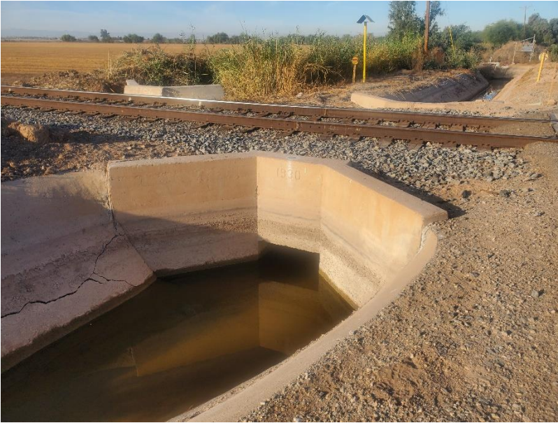
Figure 6: Overview of Niland to Calexico Railroad and culvert undercrossing dated to 1930 at north end of Project area, facing southwest.
