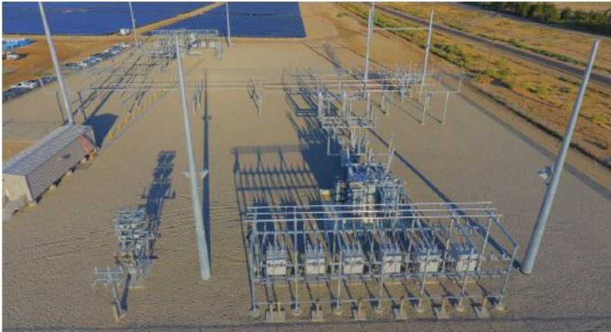
Figure 2-6. Representative Example of Typical Substation Design
