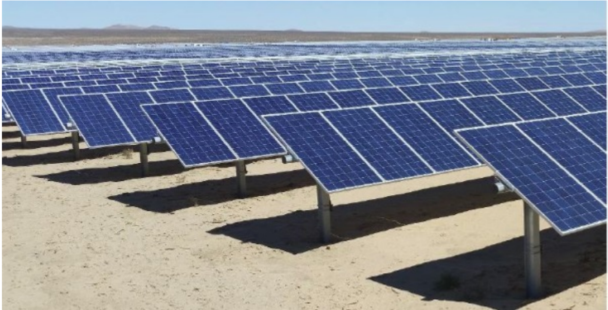
Figure 2-5. Representative Example of Typical Single-Axis Tracking Solar Panels
