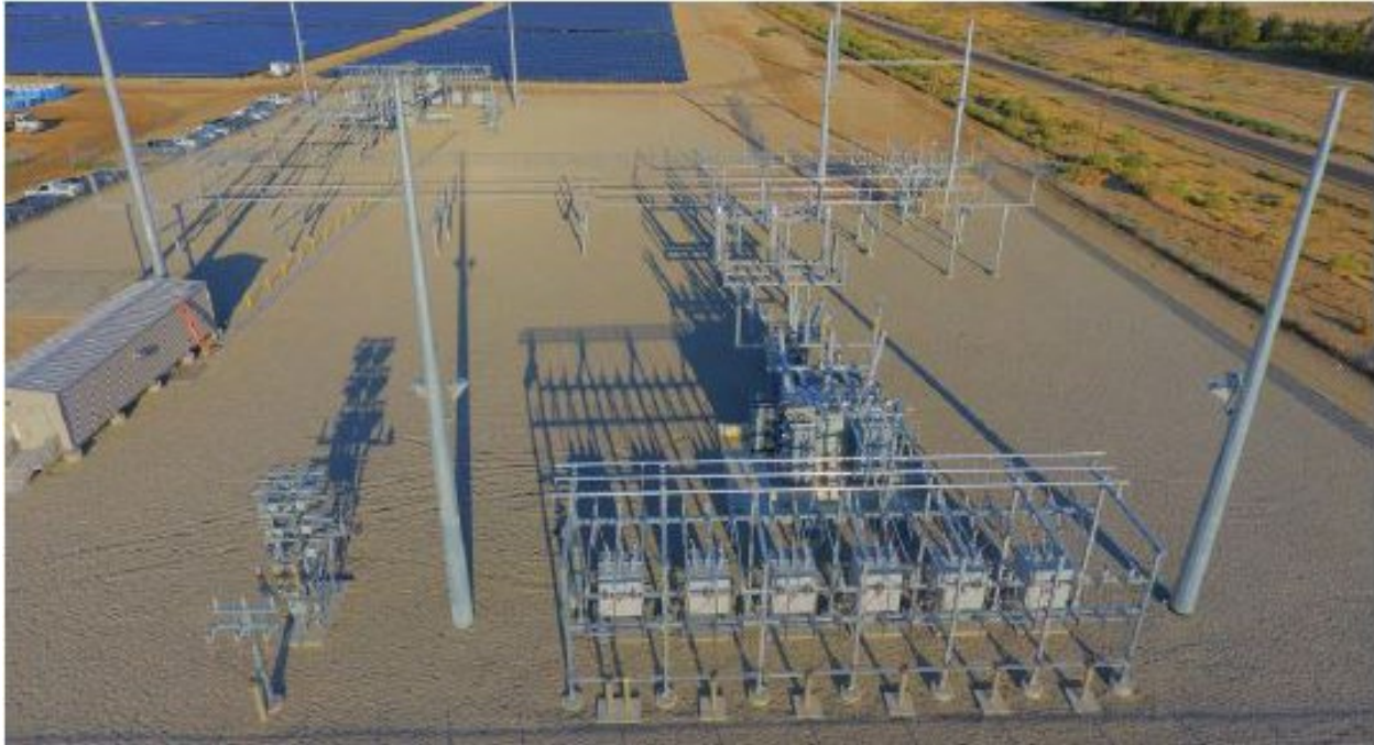
Figure 2-6. Representative Example of Typical Substation Design
