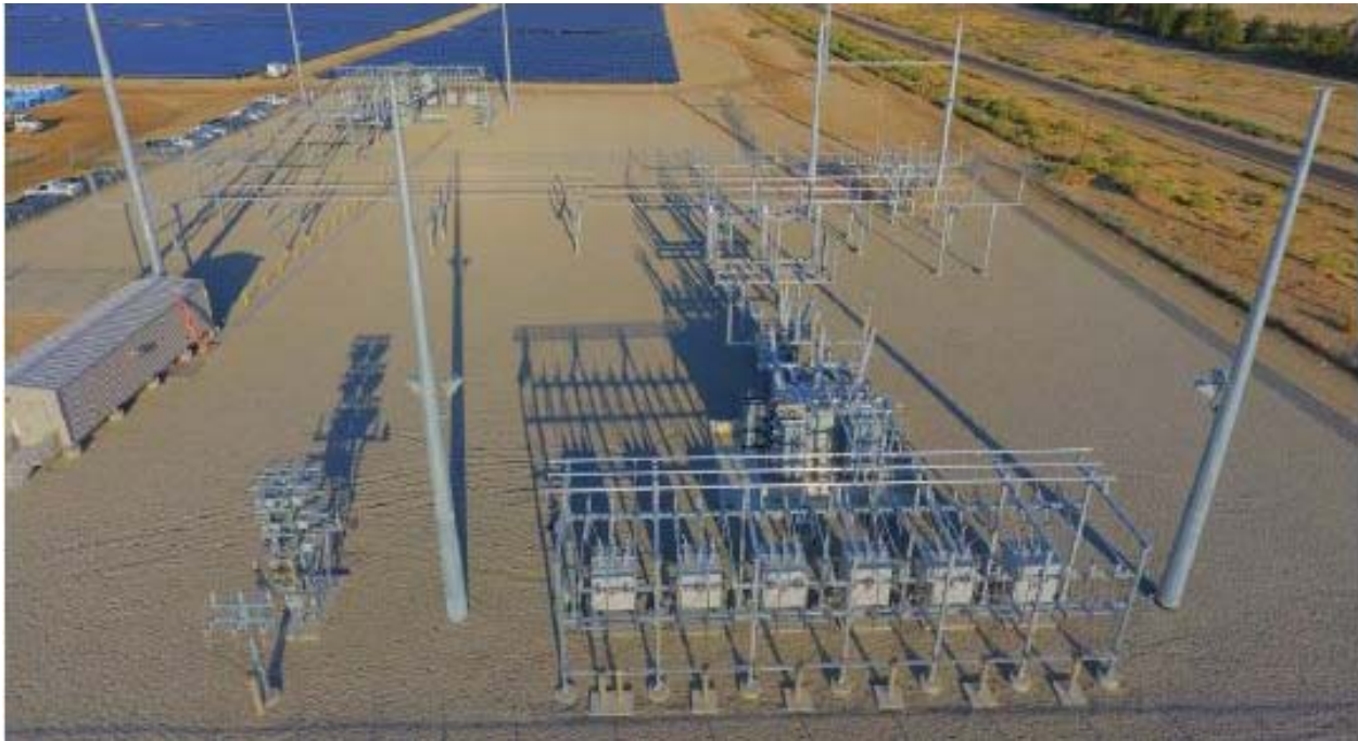
Figure 3-6. Representative Example of Typical Substation Design
