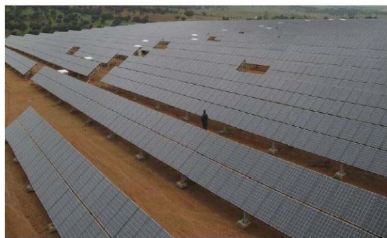
Typical Fixed-Tilt Solar Panel Rows
