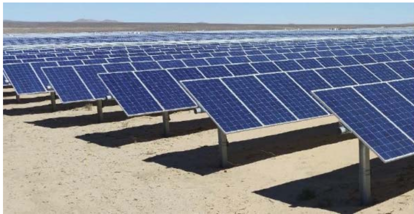
Typical Single-Axis Tracking Solar Panels
