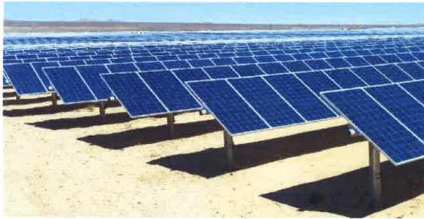
Typical Single-Axis Tracking Solar Panels
