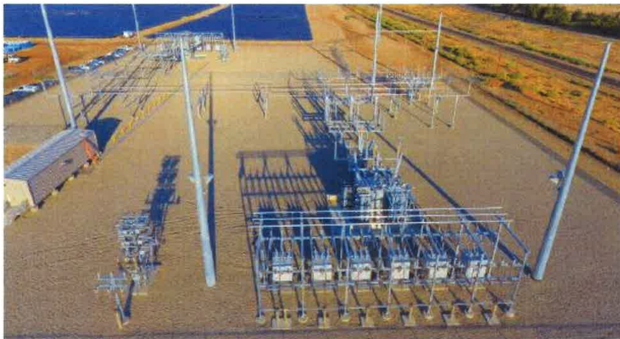
Figure 3-6. Representative Example of Typical Substation Design
