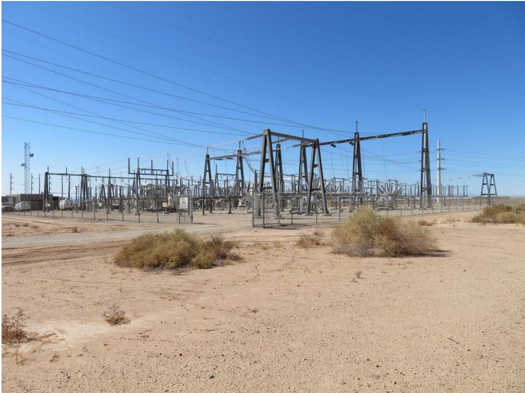
Photo 7: West-facing view of the Midway Substation.
