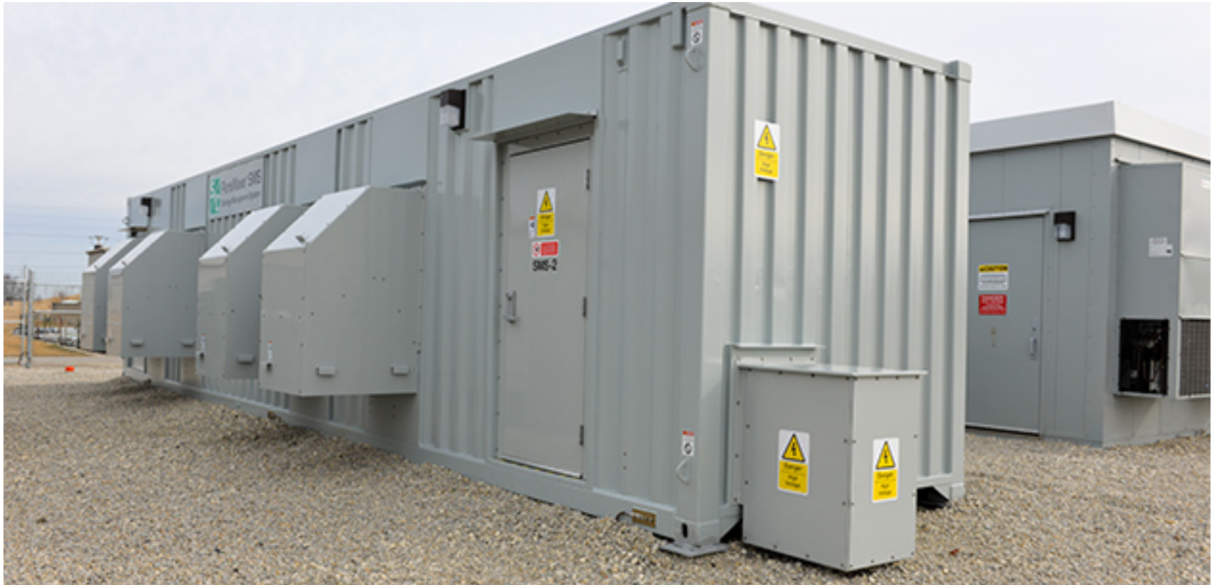
Figure 3-6. Typical Battery Storage Container
