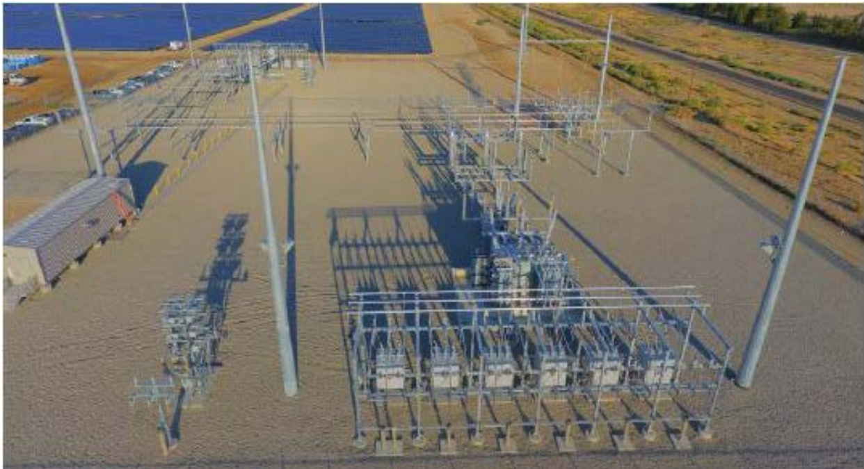
Figure 3-5. Representative Example of Typical Substation Design
