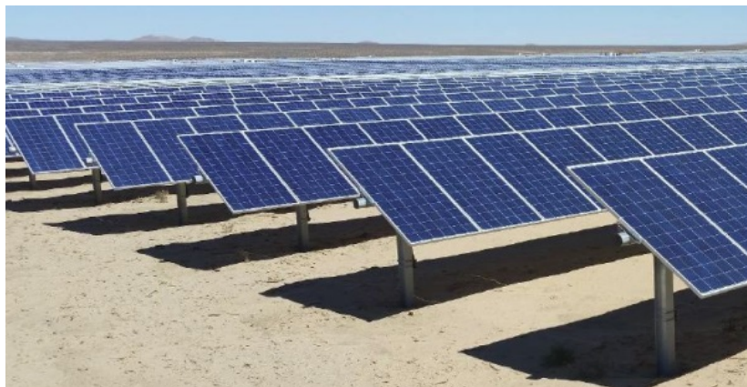
Figure 3-4. Representative Example of Typical Single-Axis Tracking Solar Panels
