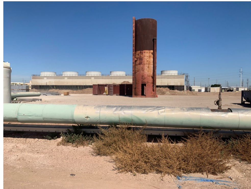
Photo 4: Proposed geothermal facility area looking north from the middle of the southern edge. Existing cooling towers in background.
