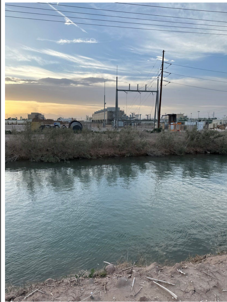
Photo 18: Existing Heber substation and transmission line located adjacent to the proposed geothermal facilities area.
