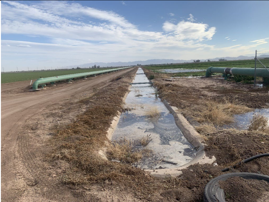
Photo 15: Concrete-lined v-ditch and existing pipeline, looking south. Proposed transmission line would be mounted to the green pipeline on the left side of the frame.
