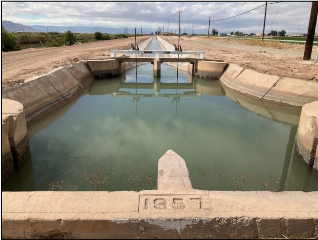
Figure 5-13. Portion of Dogwood Canal east of Pitzer Road showing concrete lining and check/drop feature with 1957 date stamp, facing east
