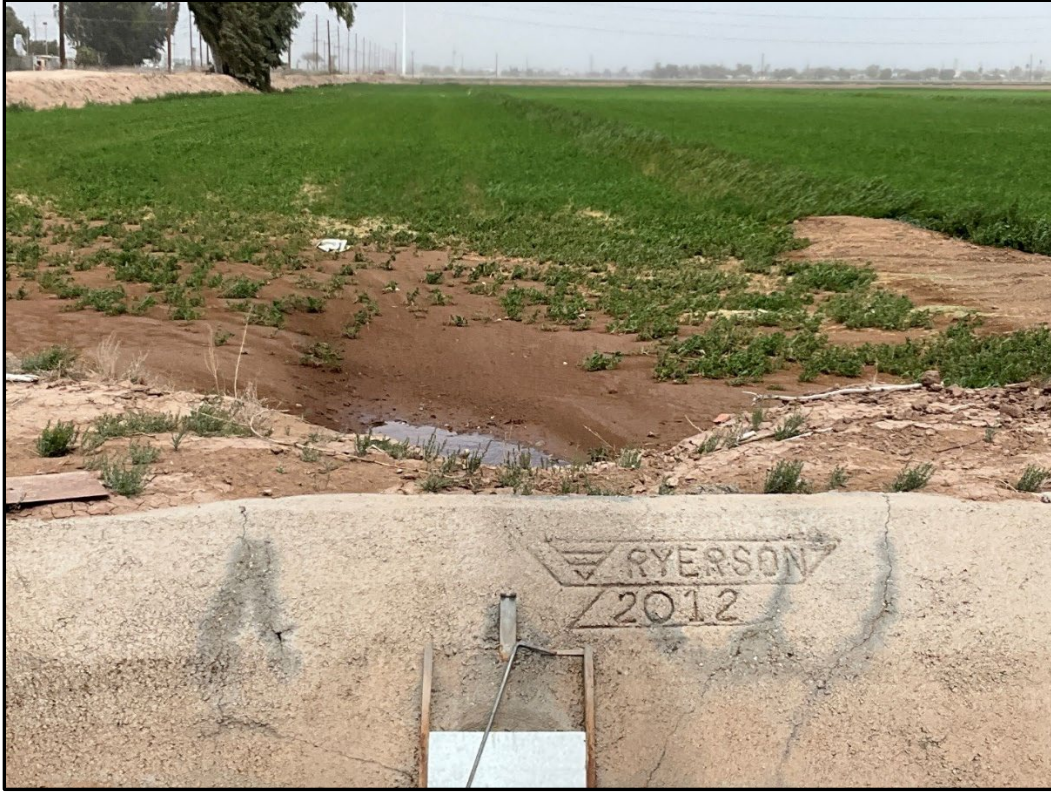
Figure 5-15. Portion of Beech Canal lateral channel with 2012 concrete date stamp, facing west
