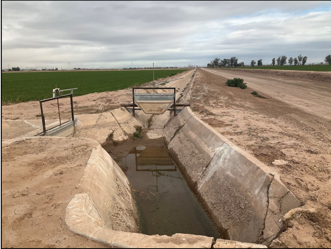
Figure 5-14. Beech Canal lateral between agricultural fields in the proposed brine pipeline alignment, facing north
