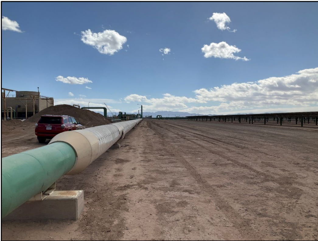
Figure 5-4. Overview of portion of brine pipeline alignment west of the HGEC facility, facing south
