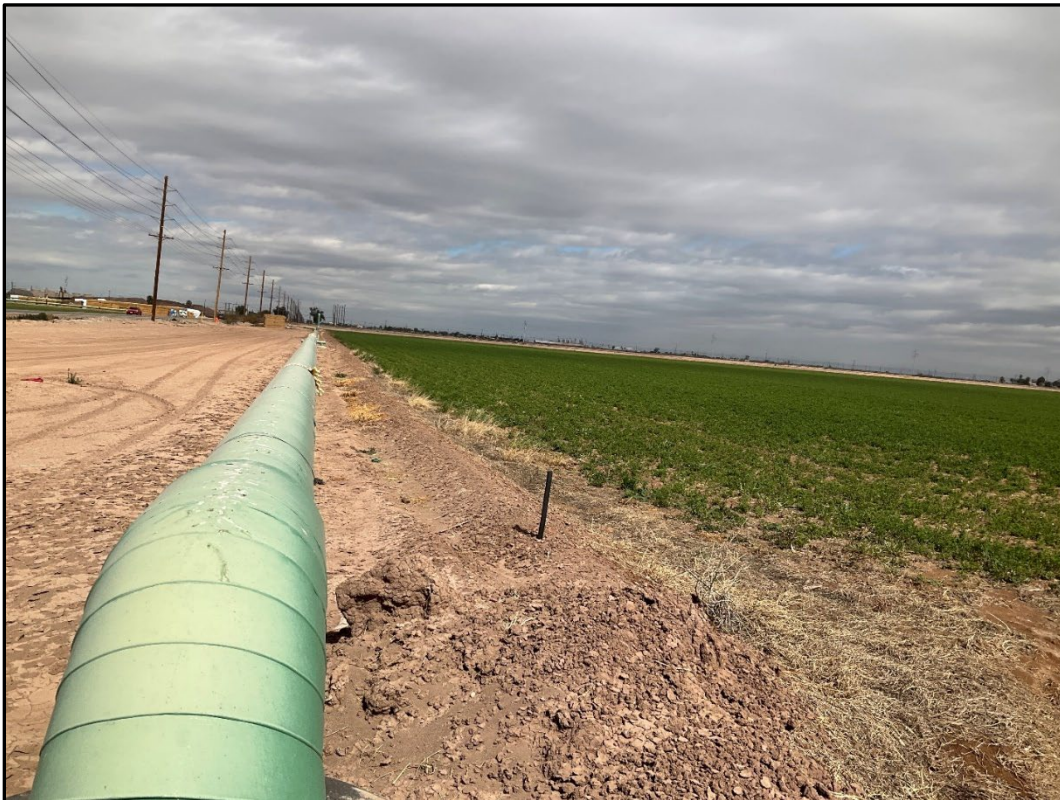
Figure 5-2. Overview of brine pipeline alignment south of the CM Canal, facing north
