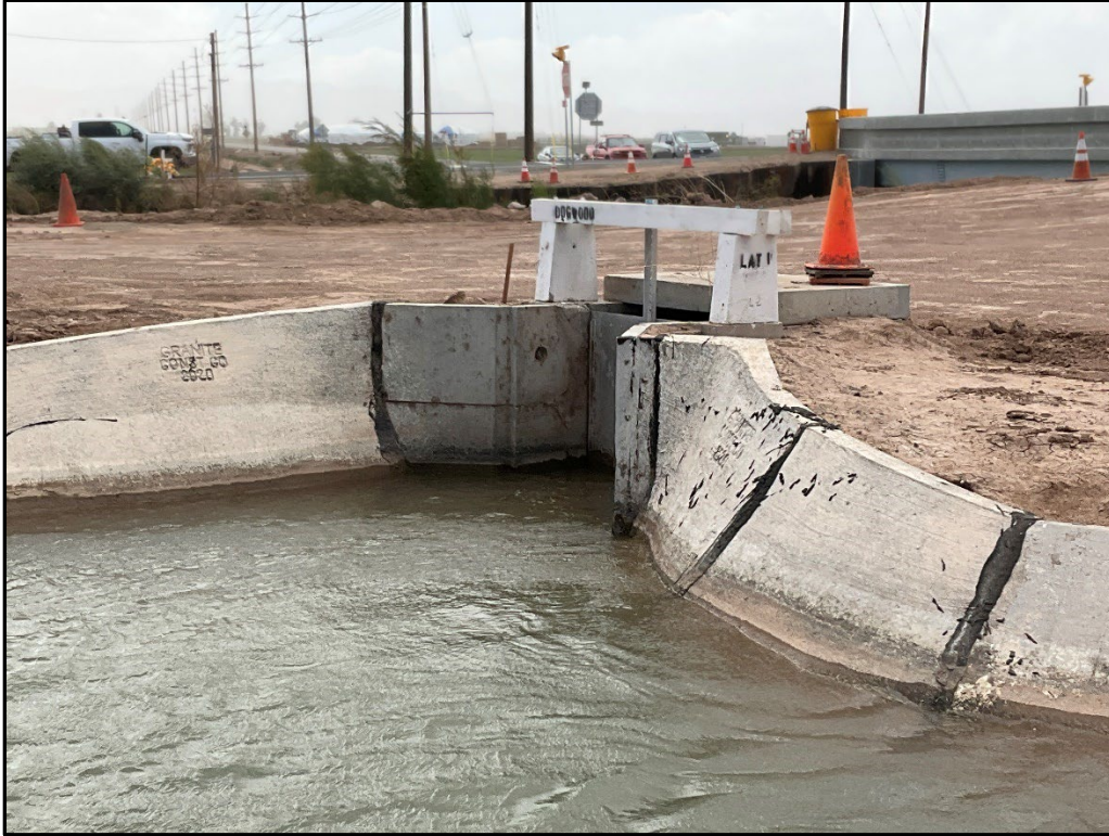
Figure 5-12. Portion of Dogwood Canal gate feature and concrete lining with date stamp, east of Dogwood Road, facing south
