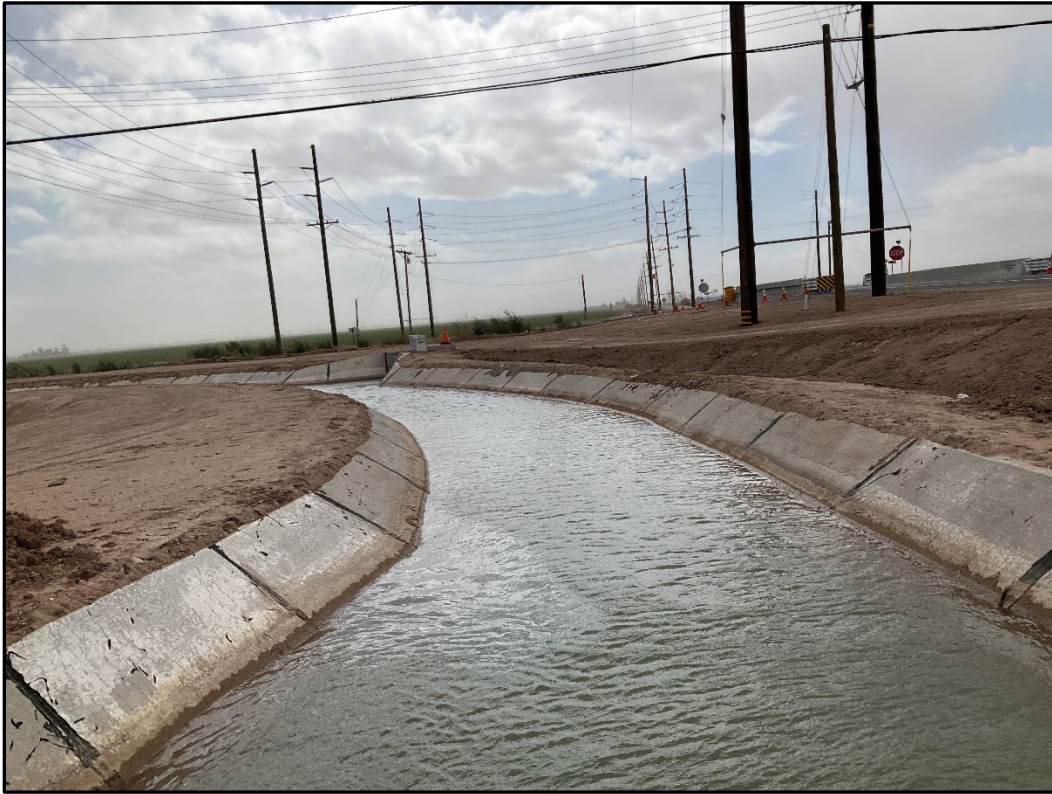
Figure 5-11. Portion of Dogwood Canal by Dogwood Road showing recently installed concrete lining, facing south
