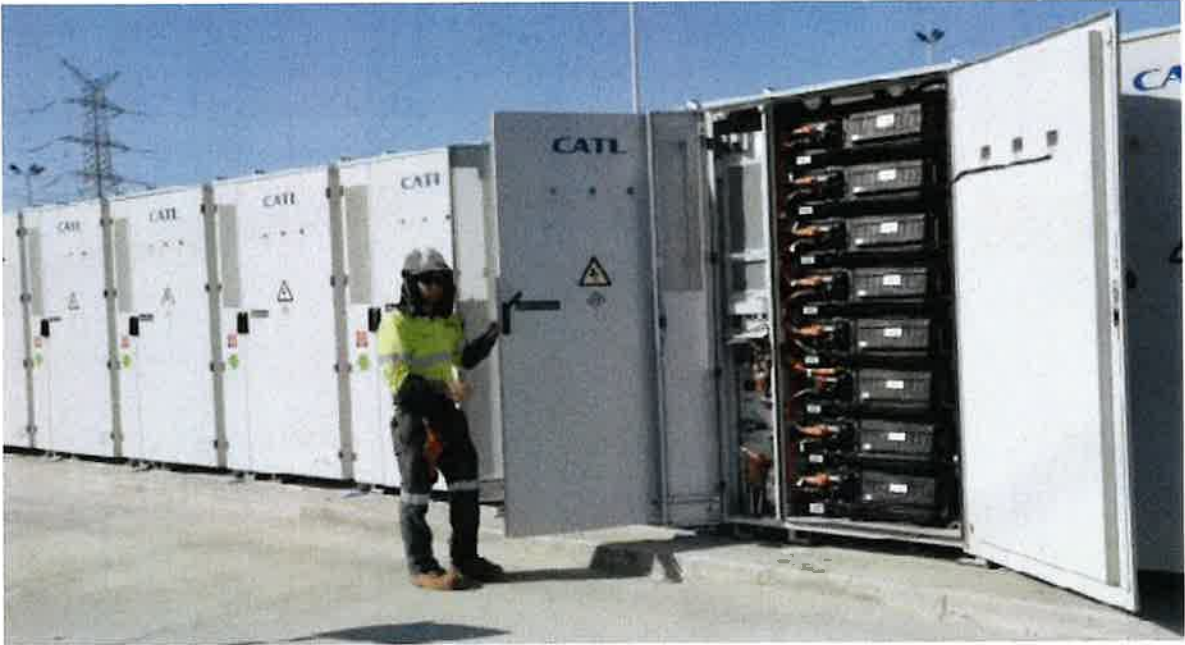
Interior of typical battery container showing small battery blocks
