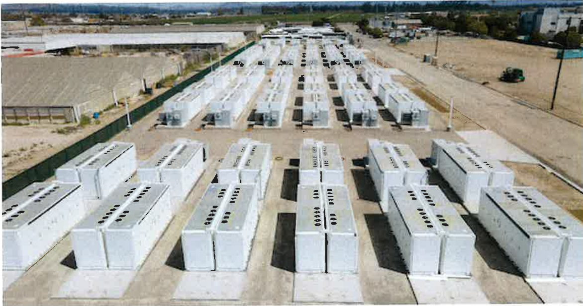
Another aerial photo of a typical BESS installation
