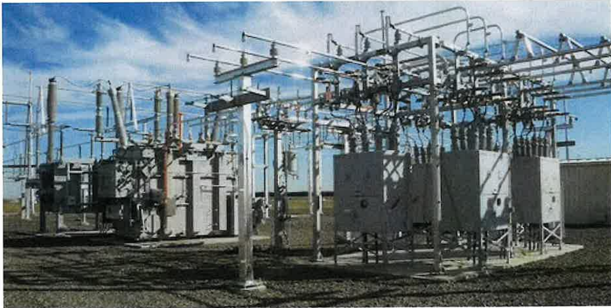
A typical small 34.5 kV – 230 kV substation
