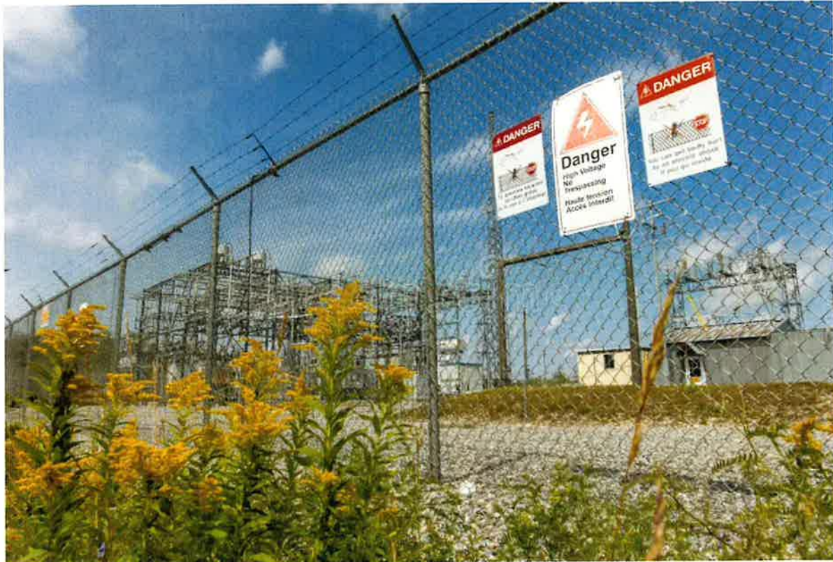
Typical fence for power generation facilities
