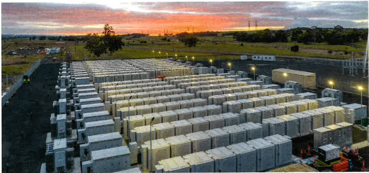
Typical BESS configuration with battery containers in the center and inverters and transformers around the perimeter
