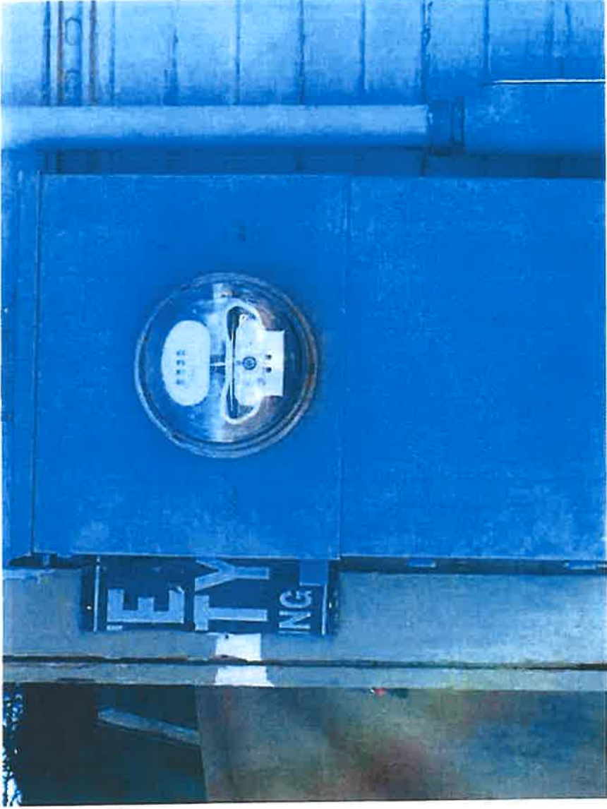
056-273-001 ELECTRIC METER SAB 01-11-21
