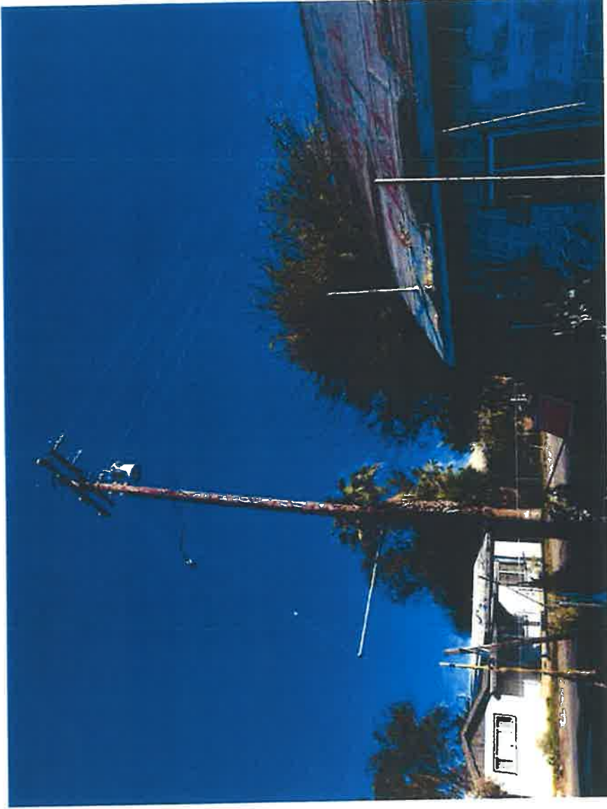
056-273-001 IID TRANSFORMER AND SERVICE ON SIDE OF THE HOUSE SAB 01-11-21
