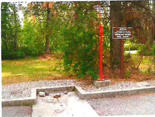
Sani dump with rinse water - not drinkable water
