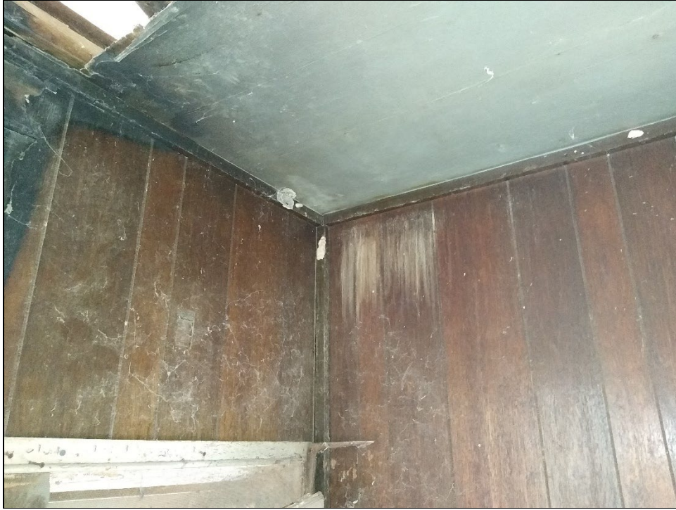
Photo 13: Interior of bat roost building, guano and staining visible.
