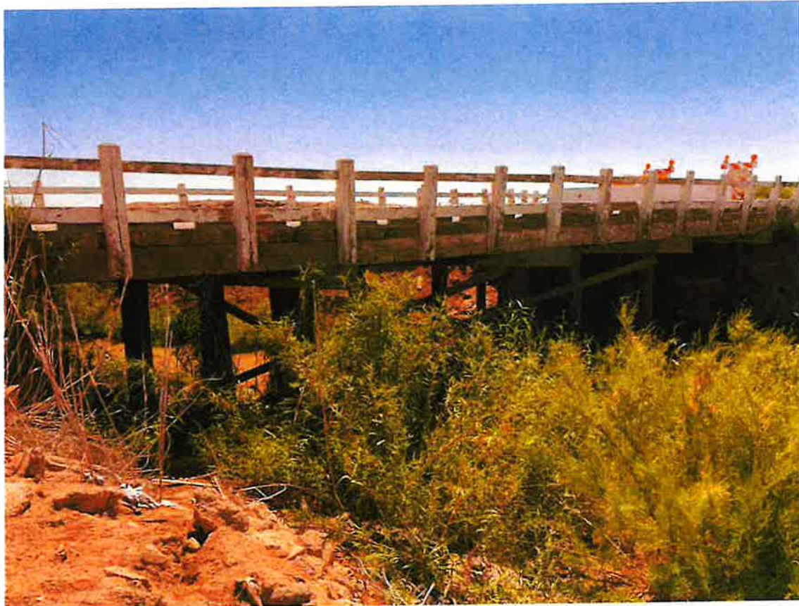
Photograph 4: Overview of the bridge from the north bank of the Central Drain Canal. View southeast, April 2, 2024.
