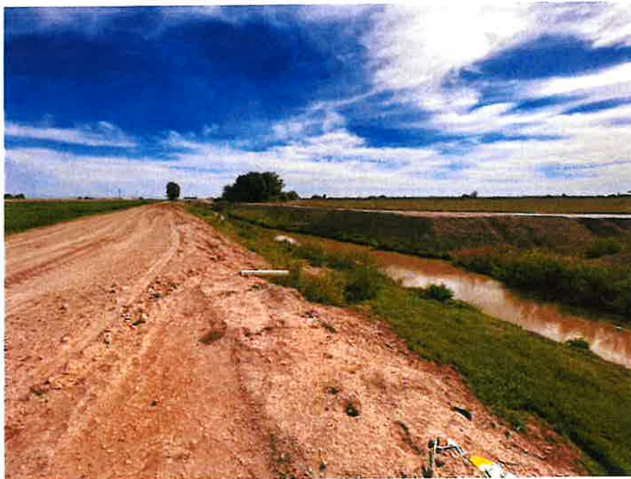
Photograph 2: Overview of the Central Drain Canal at Meloland Road. View northeast, April 2, 2024.
