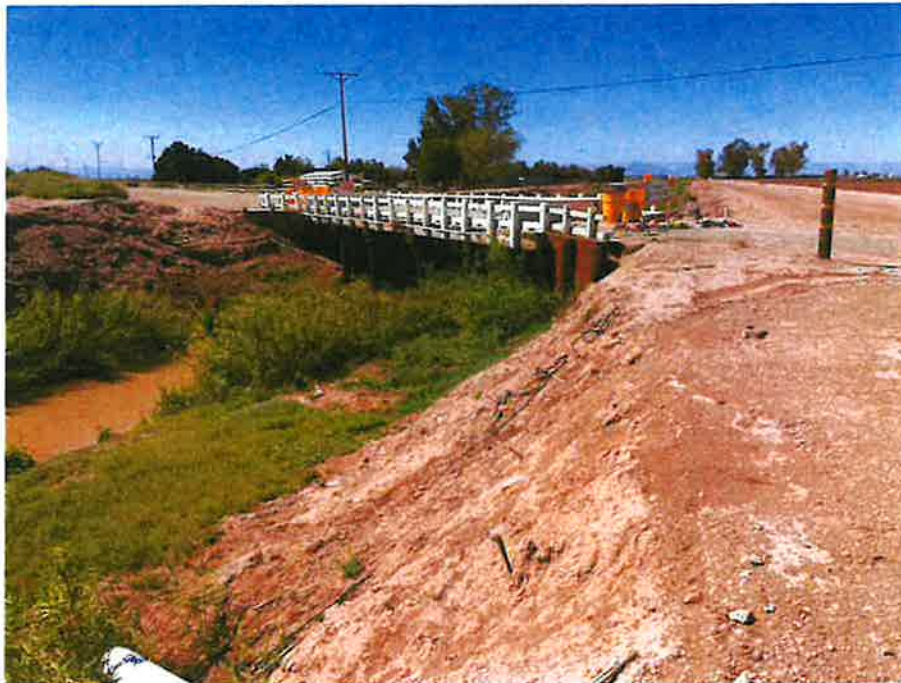
Photograph 1: Overview of the Meloland Bridge (No. 58C-0155) over the Central Drain Canal. View southwest, April 2, 2024.
