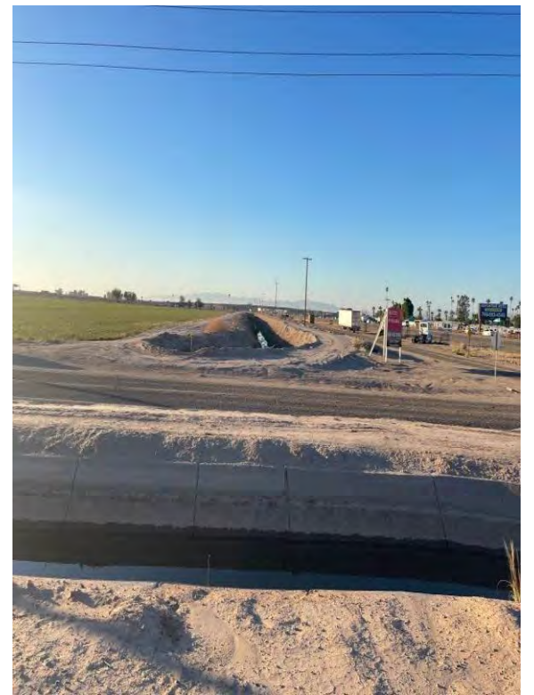
12. Acacia Canal, Ross Road, site, Acacia Drain, Hawes Road, SR 111 and RV Park looking south
