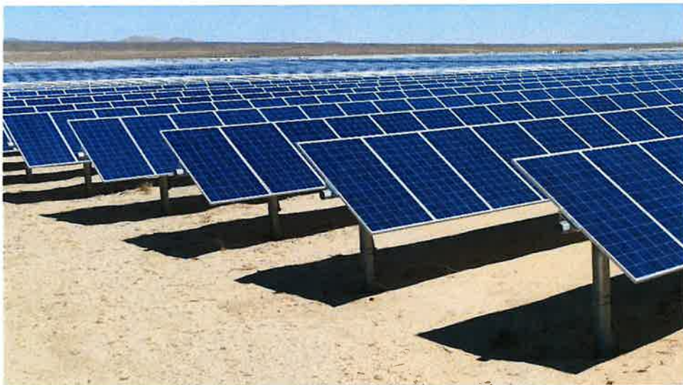
Typical single axis tracking solar panels
