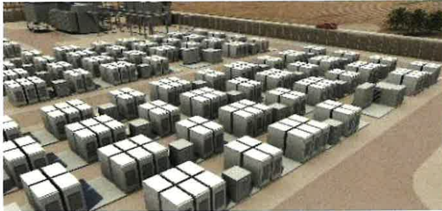
Modular BESS Installed on Multiple Concrete Pads
