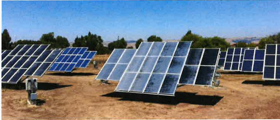
Typical dual axis tracking solar panels
