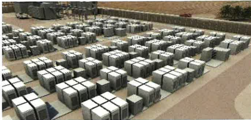
Modular BESS Installed on Multiple Concrete Pads
