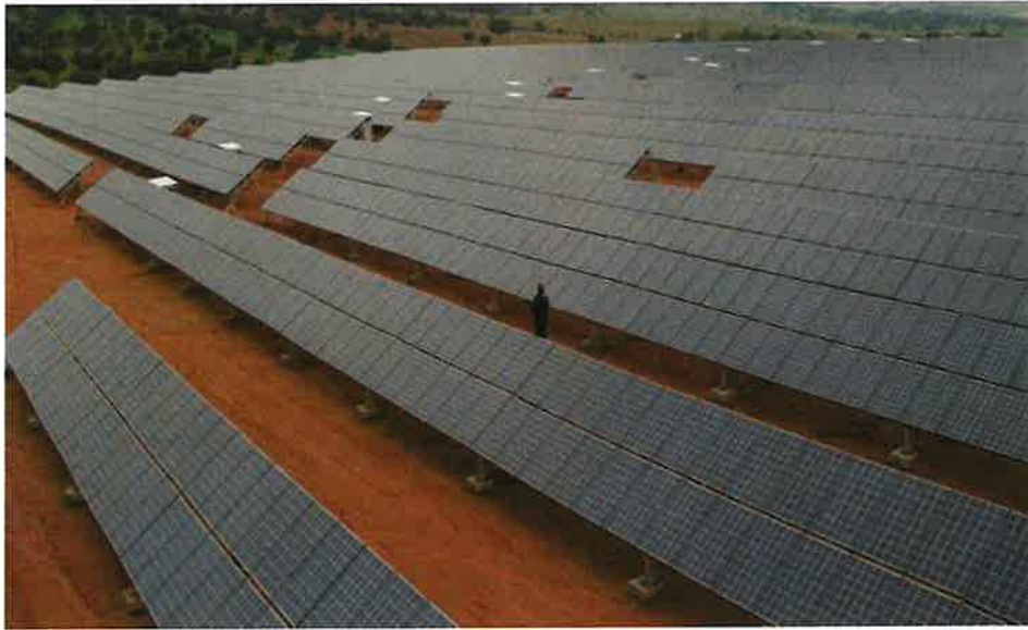
Typical fixed-tilt solar panel rows
