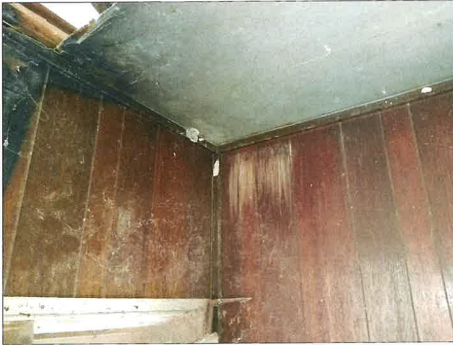
Photo 13: Interior of bat roost building, guano and staining visible.
