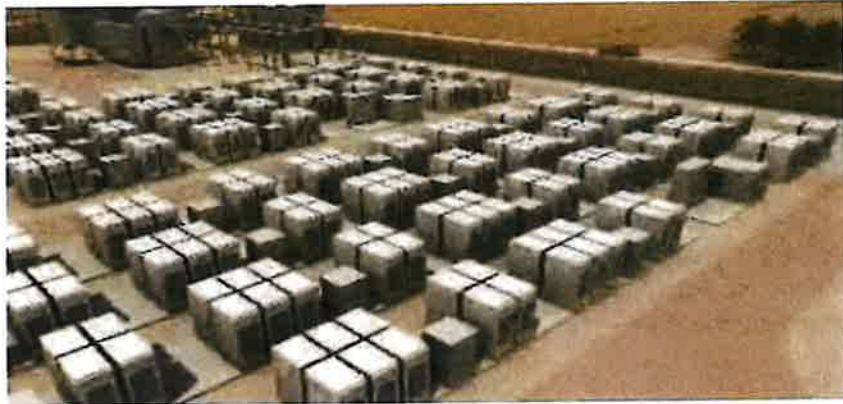
Modular BESS Installed on Multiple Concrete Pads
