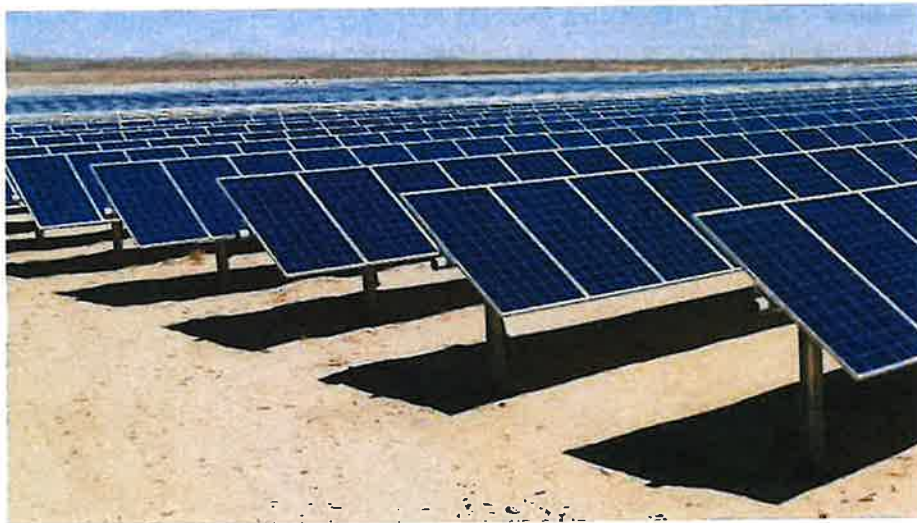
Typical single axis tracking solar panels
