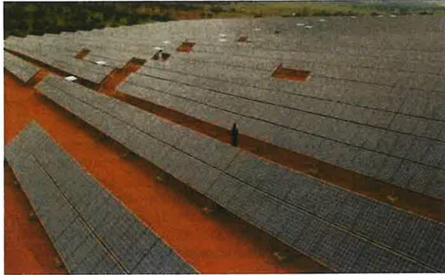
Typical fixed-tilt solar panel rows
