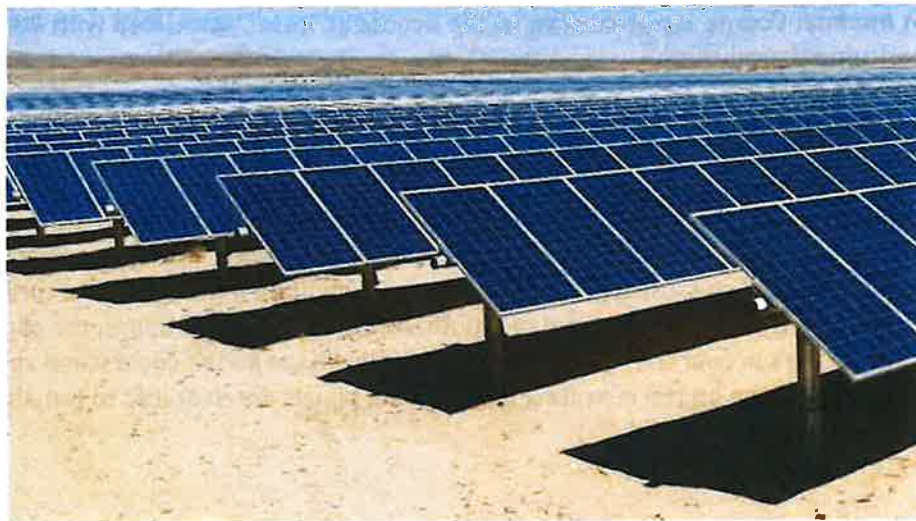
Typical single axis tracking solar panels
