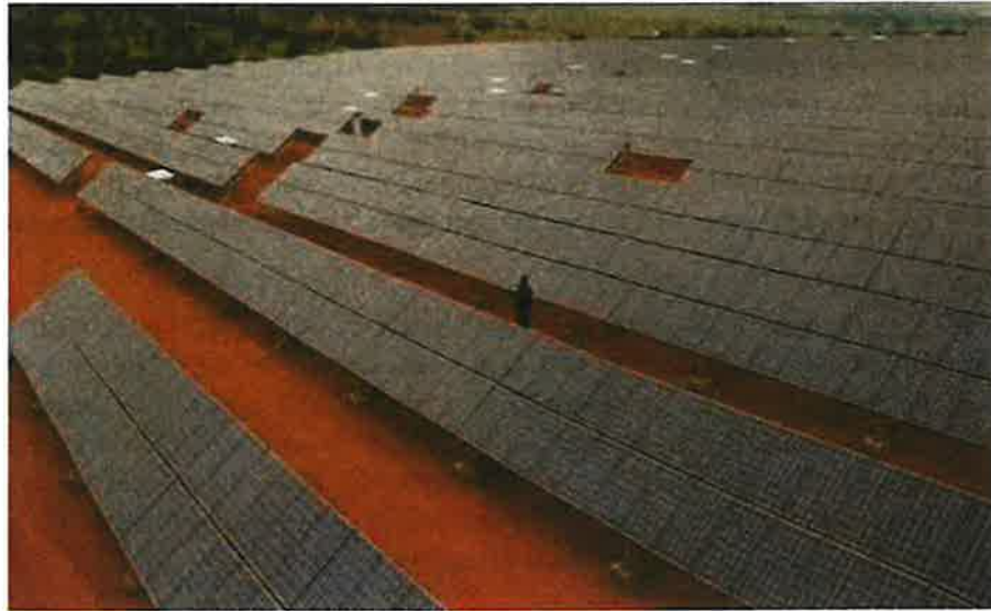
Typical fixed-tilt solar panel rows
