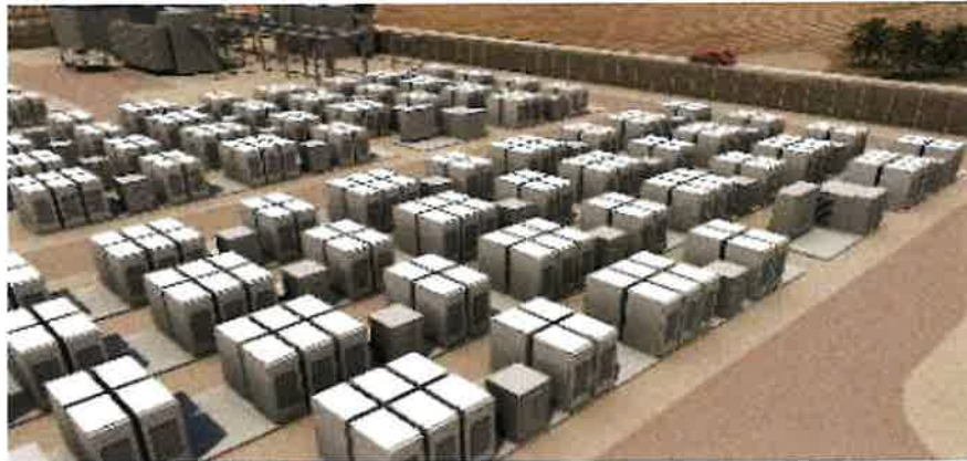
Modular BESS Installed on Multiple Concrete Pads
