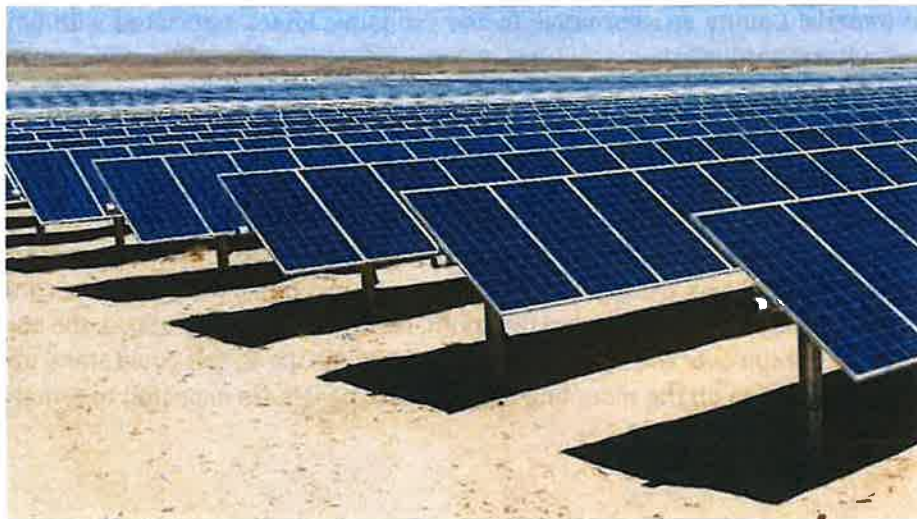
Typical single axis tracking solar panels
