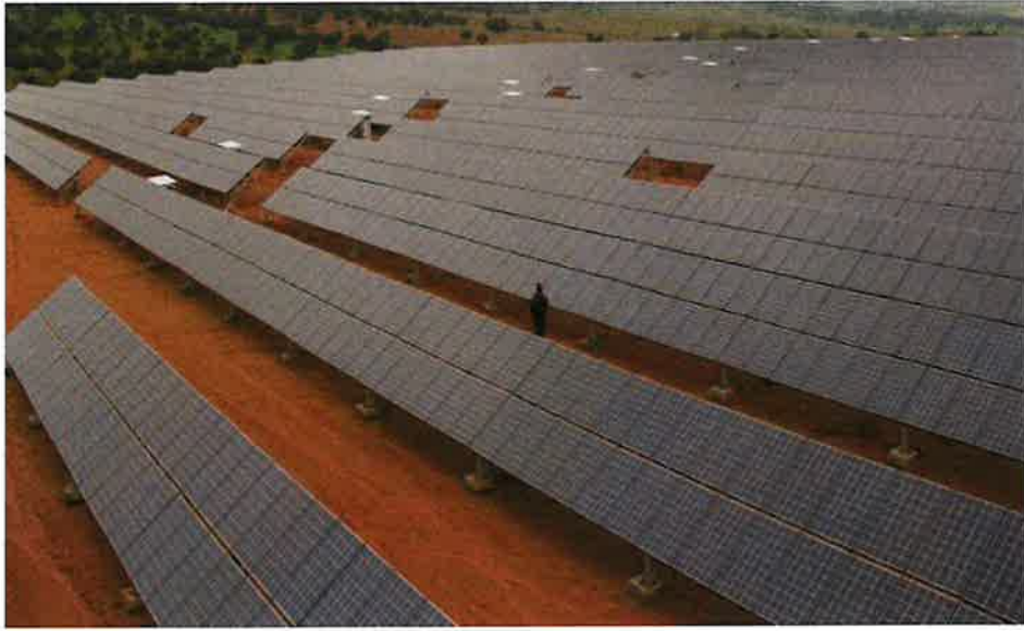
Typical fixed-tilt solar panel rows
