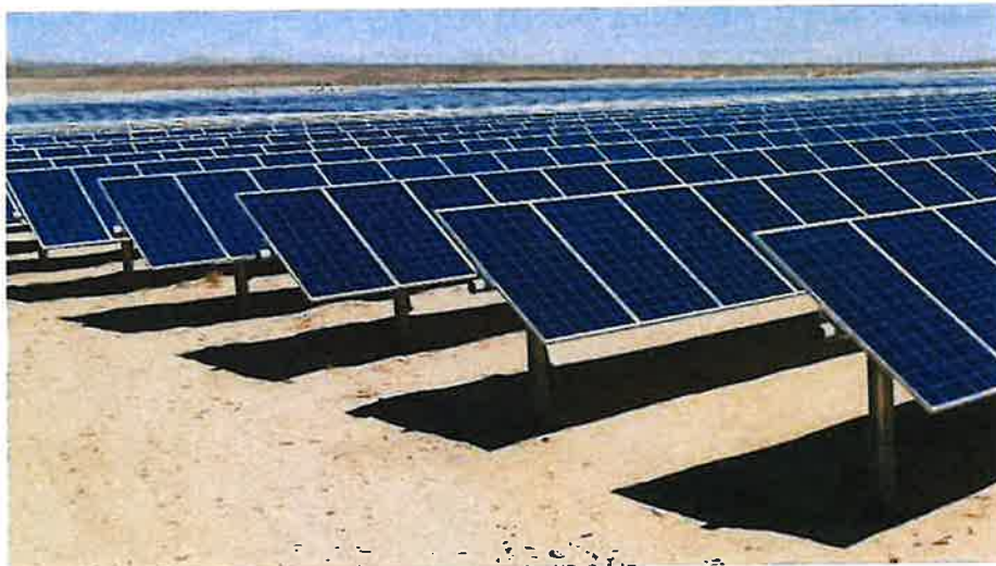
Typical single axis tracking solar panels
