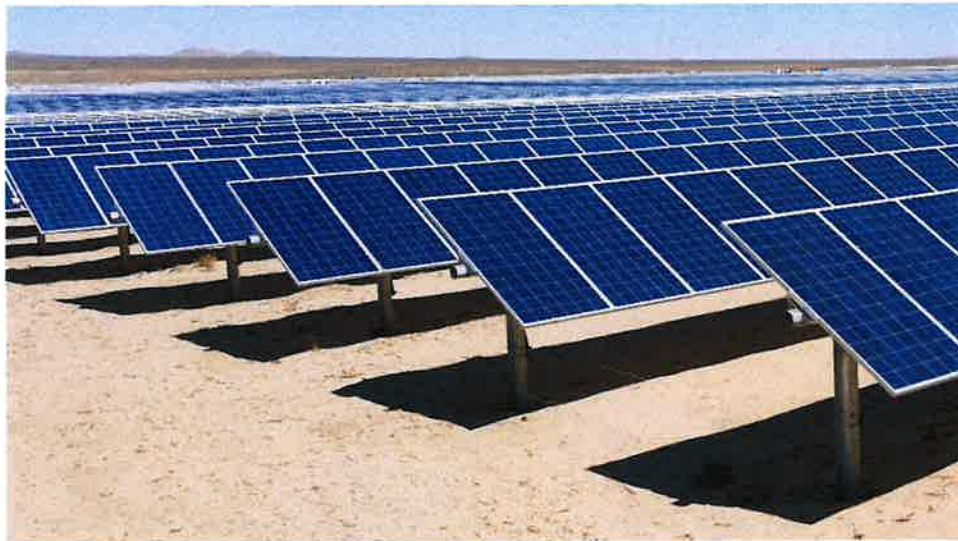
Typical single axis tracking solar panels
