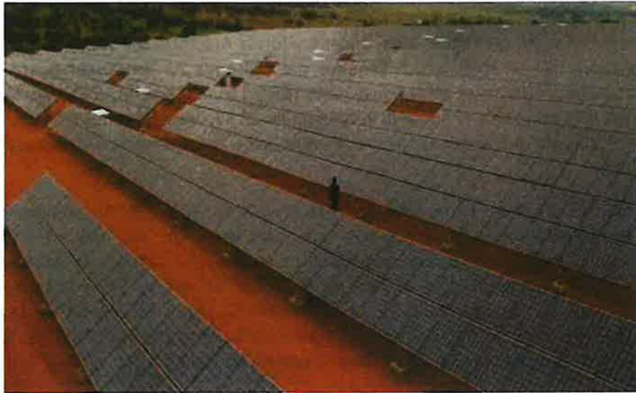
Typical fixed-tilt solar panel rows
