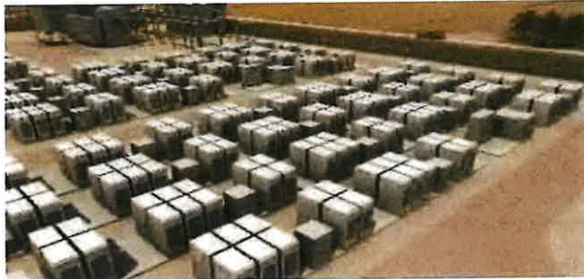
Modular BESS Installed on Multiple Concrete Pads
