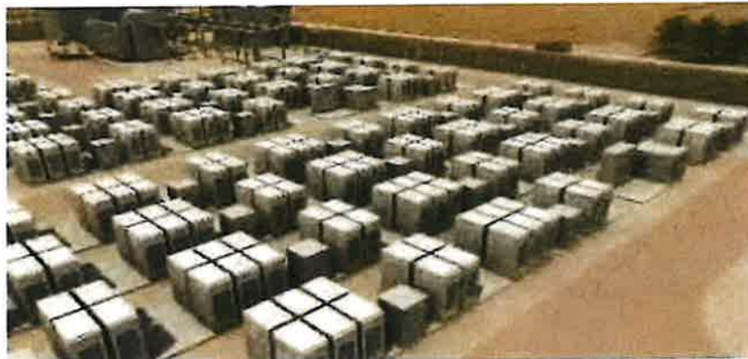
Modular BESS Installed on Multiple Concrete Pads
