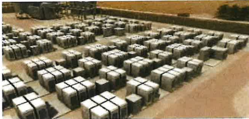
Modular BESS Installed on Multiple Concrete Pads
