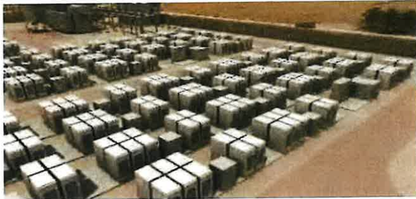
Modular BESS Installed on Multiple Concrete Pads
