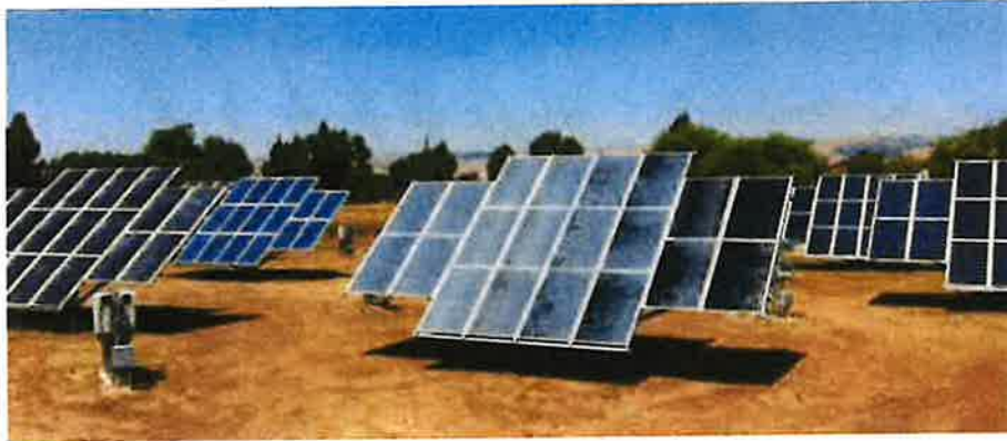
Typical dual axis tracking solar panels
