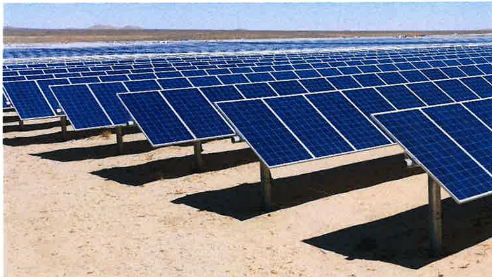
Typical single axis tracking solar panels
