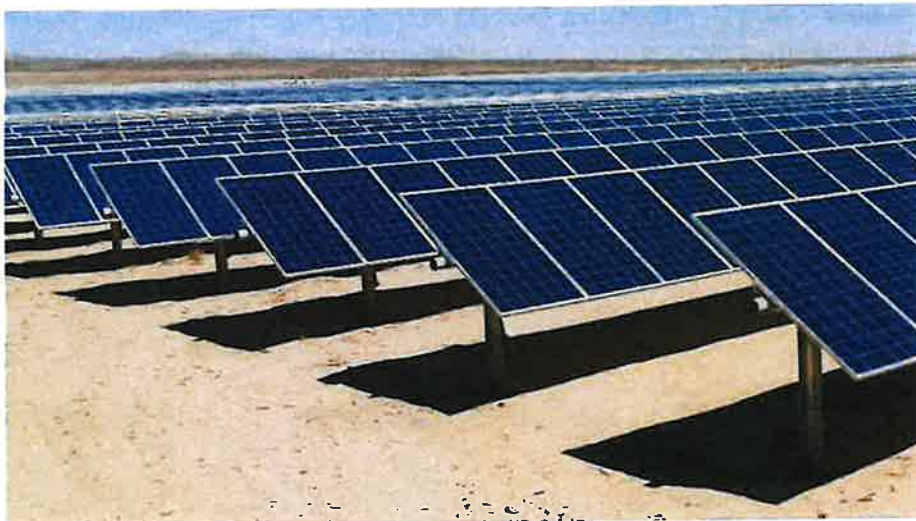
Typical single axis tracking solar panels
