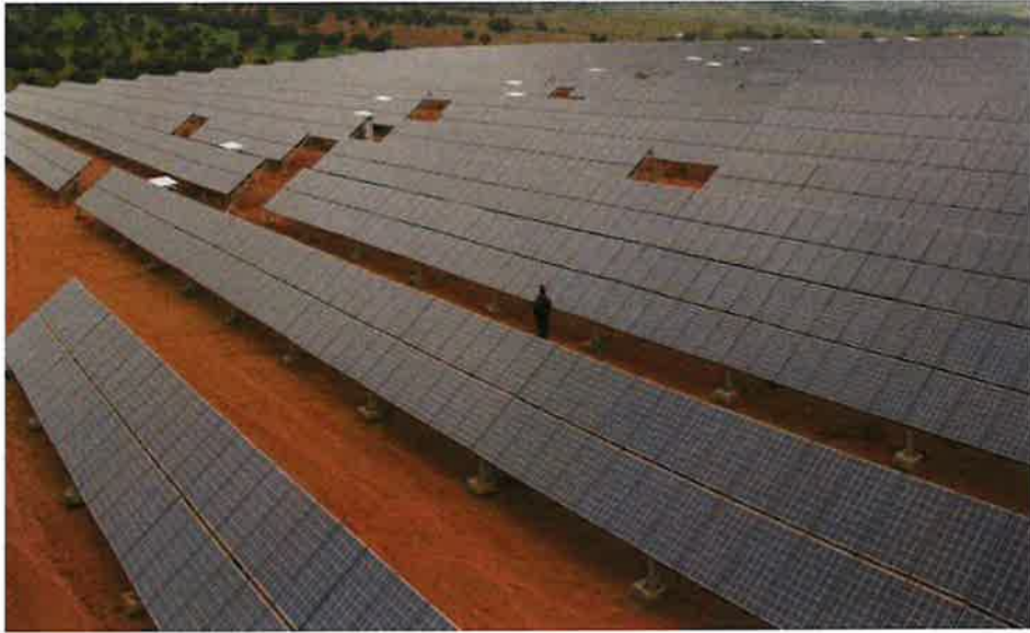
Typical fixed-tilt solar panel rows
