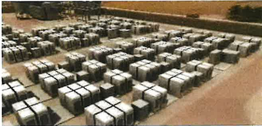
Modular BESS Installed on Multiple Concrete Pads
