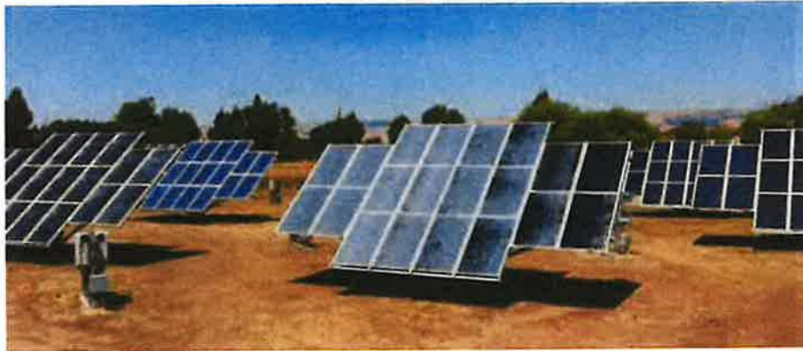
Typical dual axis tracking solar panels
