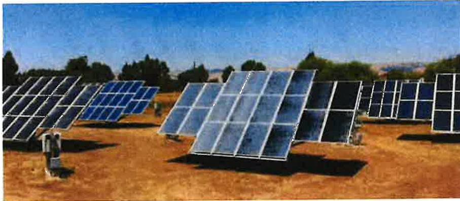
Typical dual axis tracking solar panels
