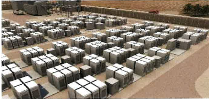
Modular BESS Installed on Multiple Concrete Pads
