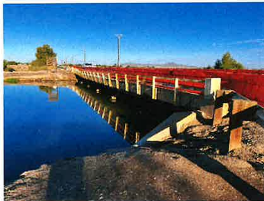
Figure 8: South side of the Picacho Bridge taken from the eastern end of the bridge, view to the west
