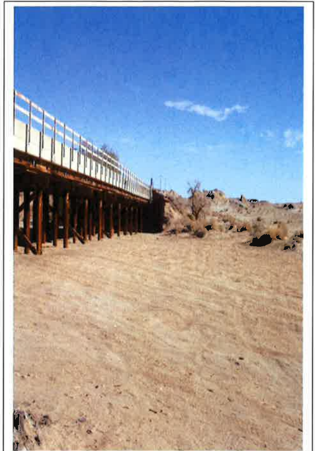
8. Bridge at south side of wash; off road vehicle road which goes under bridge
