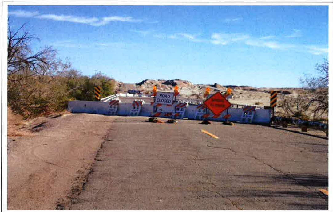
2. Evan Hewes Highway at Coyote Wash Bridge looking east; saltcedar on both sides
