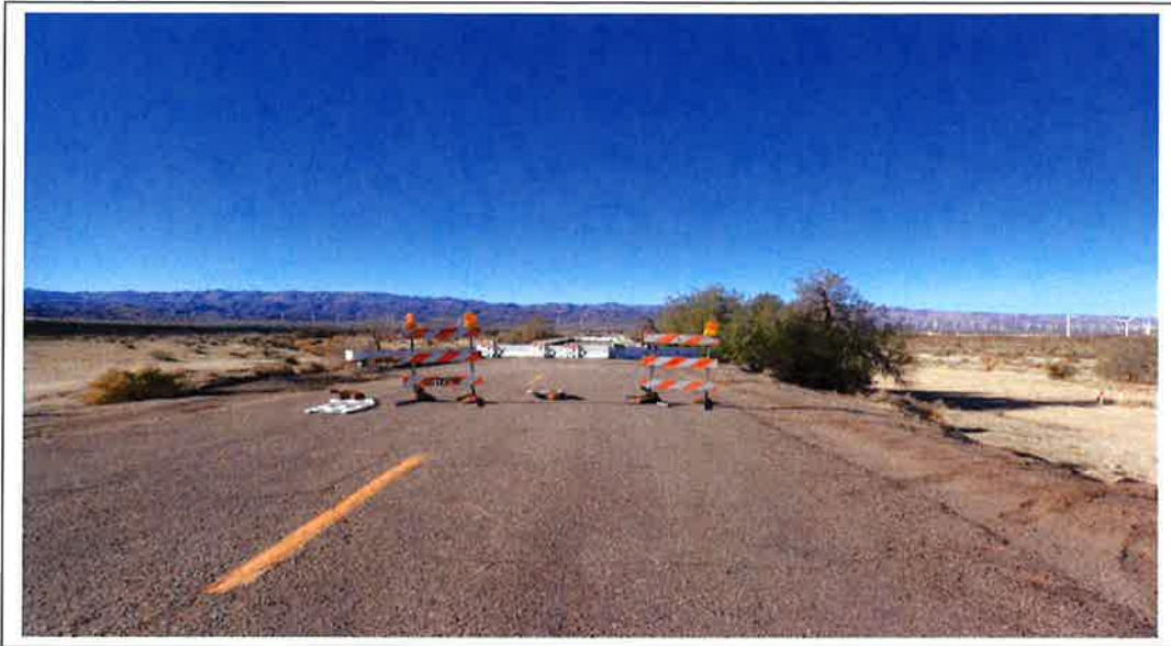
1. Evan Hewes Highway at Coyote Wash Bridge looking west; saltcedar to right
